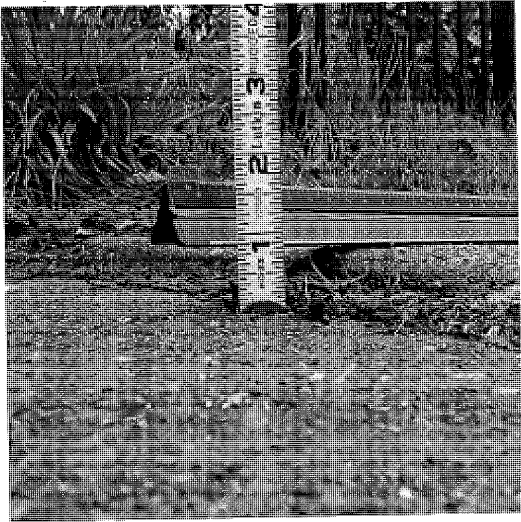
Sidewalk lifted from tree roots
